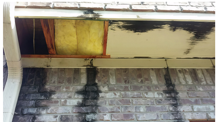
Dark honey stains, shown here on an exterior wall, can be difficult to remove. The drywall ceiling had to be replaced. Photo by Southeast Bee Removal
